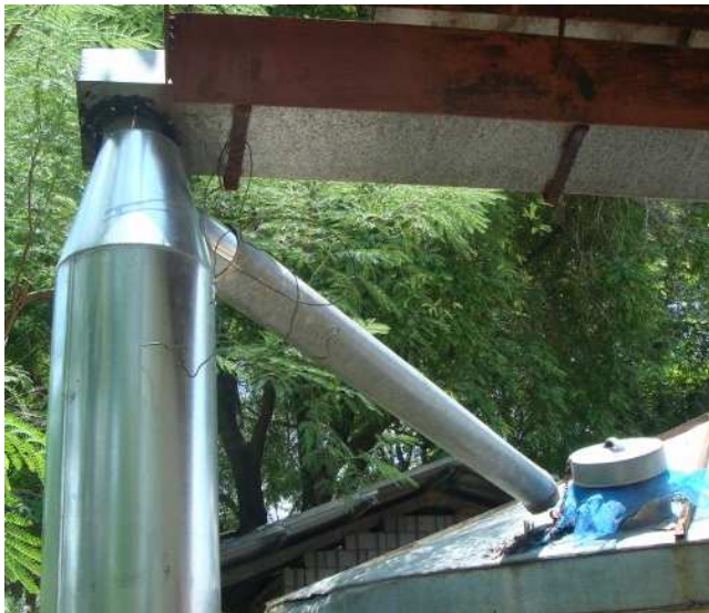
Figure 3: Connection between gutter down drain and inlet point for CP Syptin
