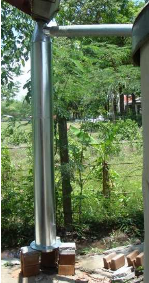
Figure 1: View of installed downspout system
